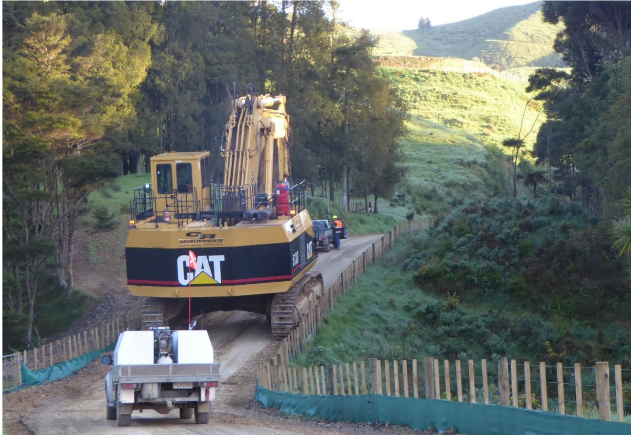
Photo 9: October 2016: 180t excavator tracking along widened farm track to gain access to the south side of the summit.
