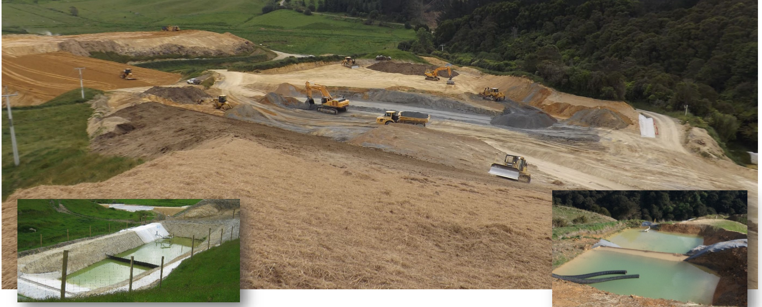
Photo 8: Area B working with varied soil conditions, including a coal seam. The area above has been stabilised to prevent erosion. (Insert: Examples of SRP's located through area B. In the background is the access track with multiple DEB's for haul road runoff control).
