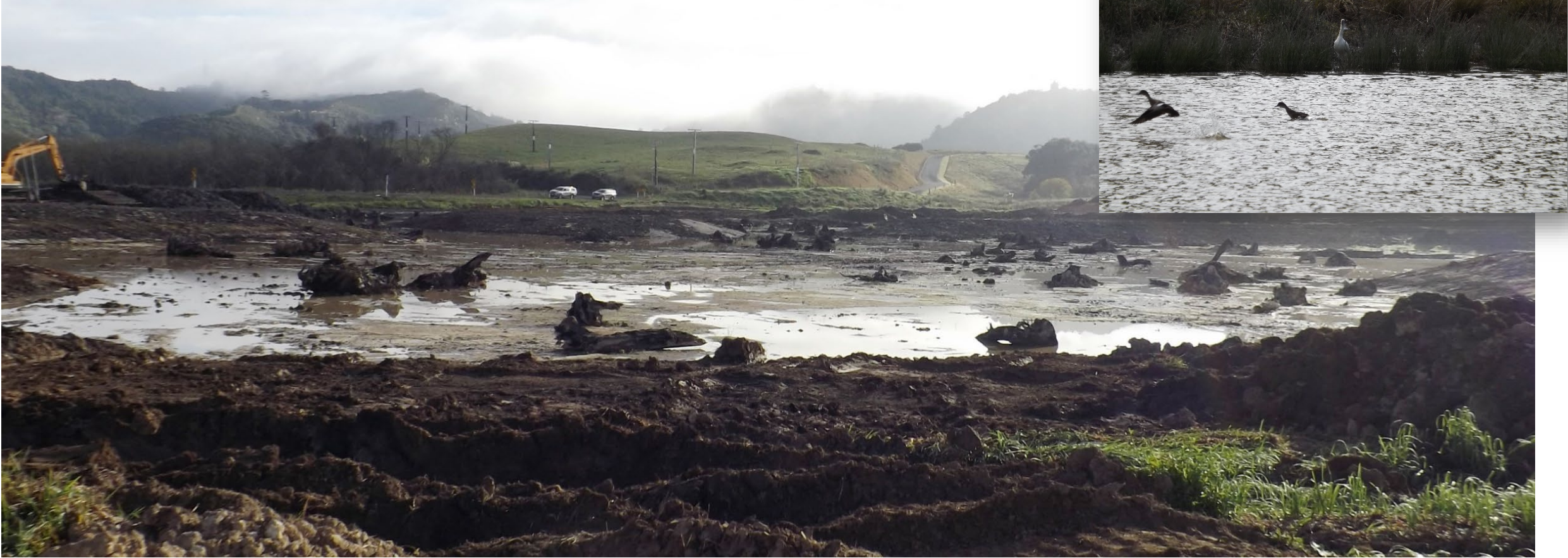
Photo 17: Evans Road wetland (5ha) under construction, which was then colonised by Royal Spoonbill, White Heron and Bittern, along with other water fowl
