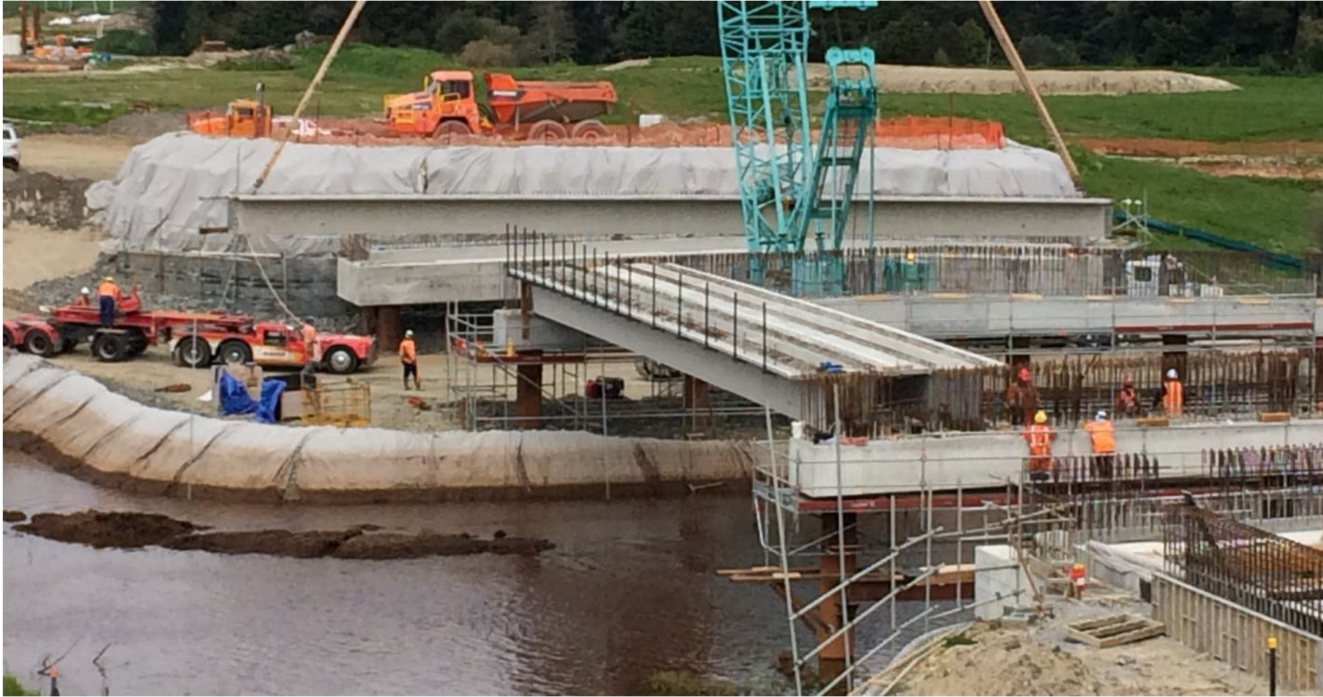
Photo 4: Bridge works over one of the Red Rivers streams (Komakorau Stream), wrapped bunds protected the stream from run-off from the crane pad. Note the water levels showing on the cloth, these river levels regularly rose to the top of the bund and there was times where it overtopped it.
