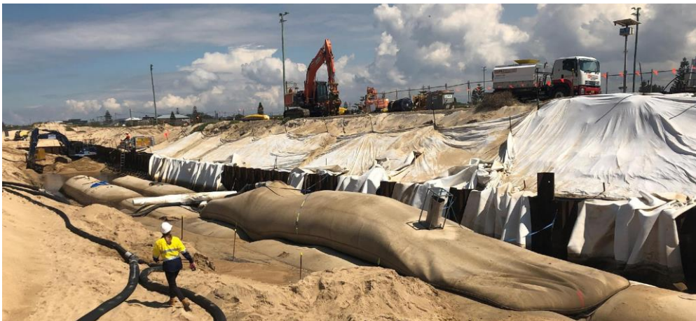
Figure 23: Natalie Patterson from Royal HaskoningDHV working on a collaborative solution to a practical design iteration at Stockton mega container site
