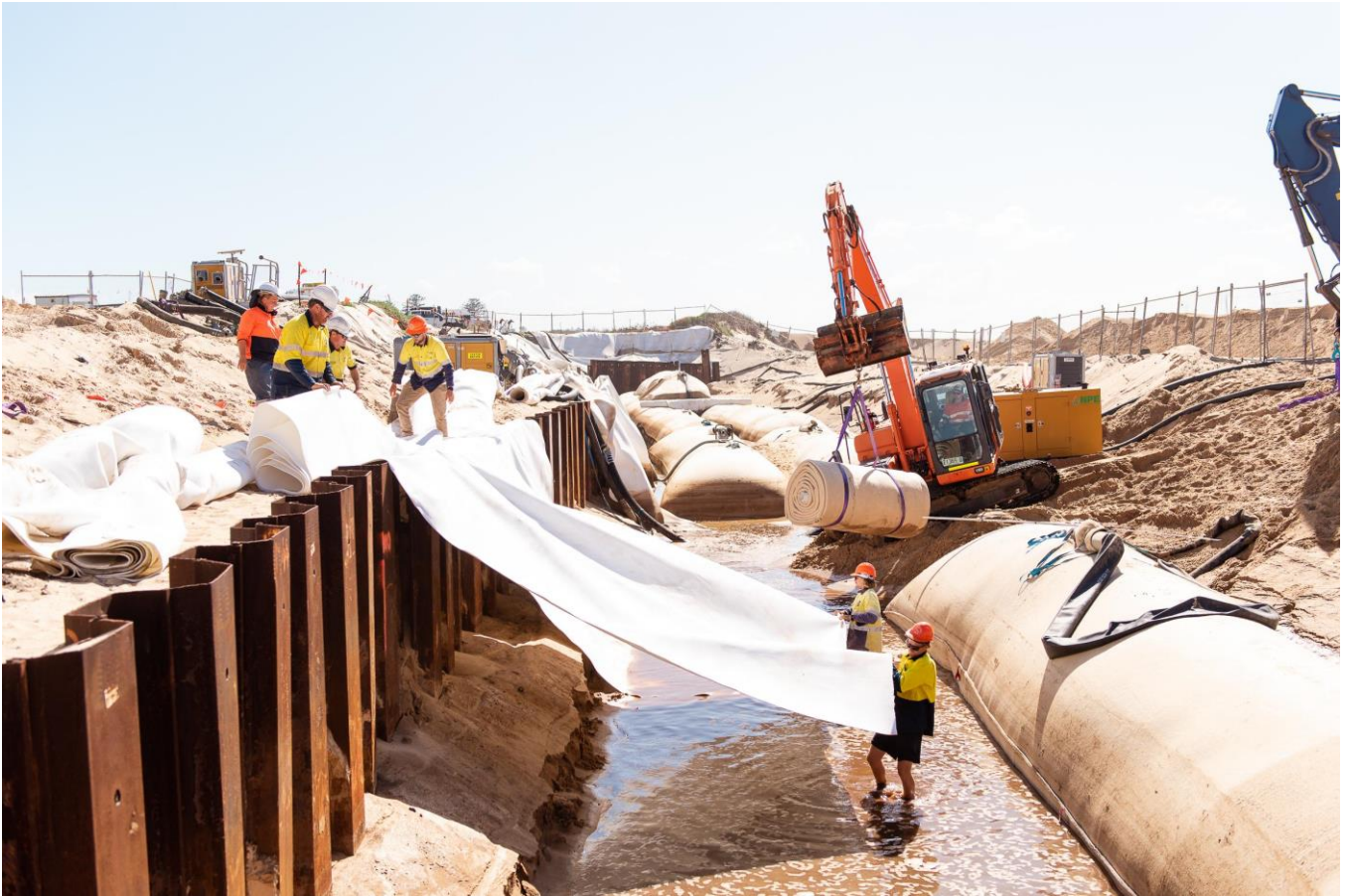
Image 2: Stockton Project team installing coastal grade geotextile to underlay mega container seawall construction.
