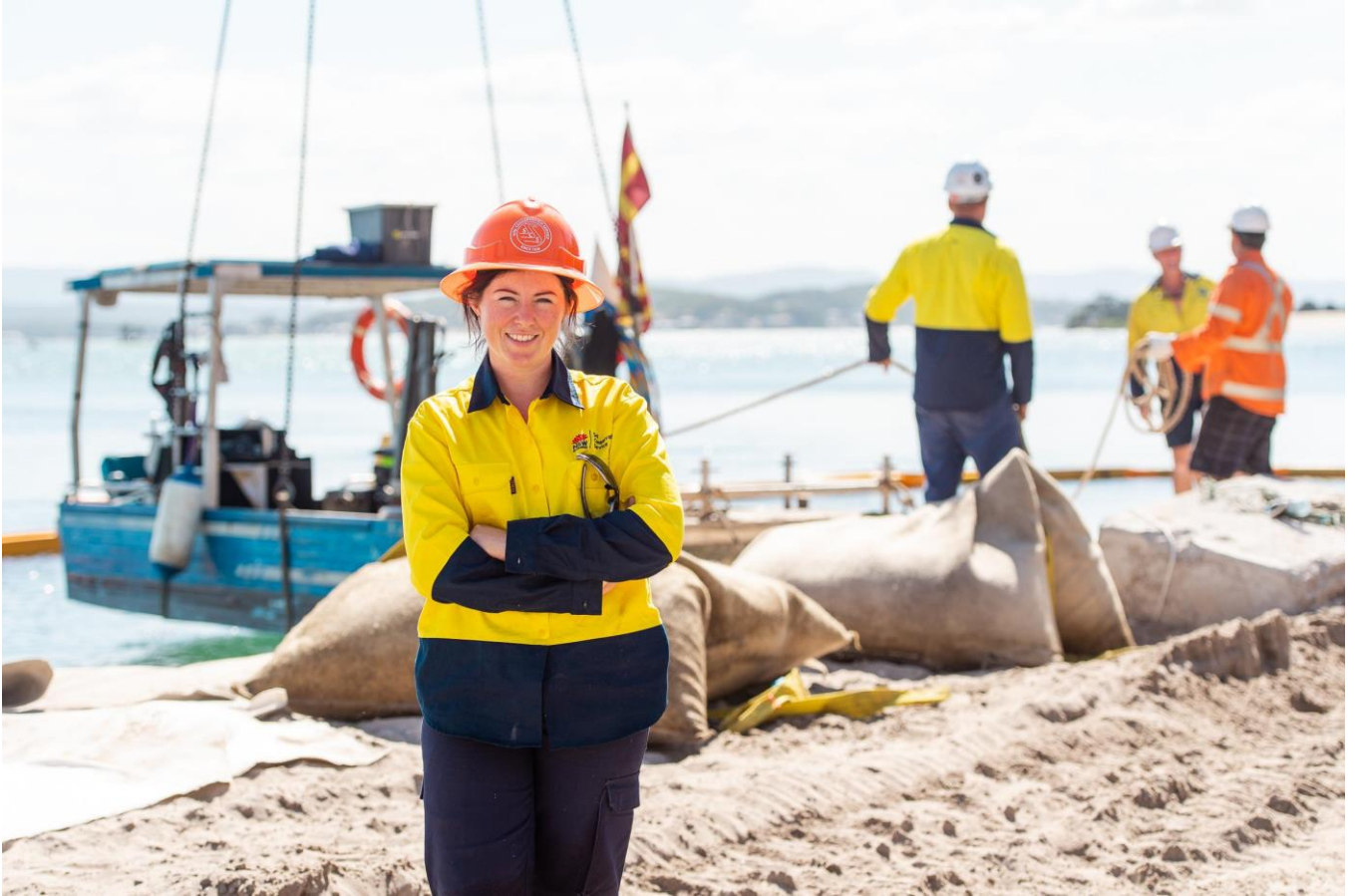
Image 1: Emma Belford from SCS ensuring the safety of the team and quality of the construction project at the Pelican Geo bag Revetment project
