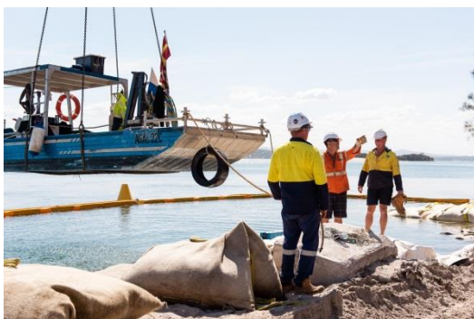
Figure 21: Rising to the challenge: Cranes, Boats, Divers, Diggers, ESC and a 1 hour construction window due to tidal exchange.
