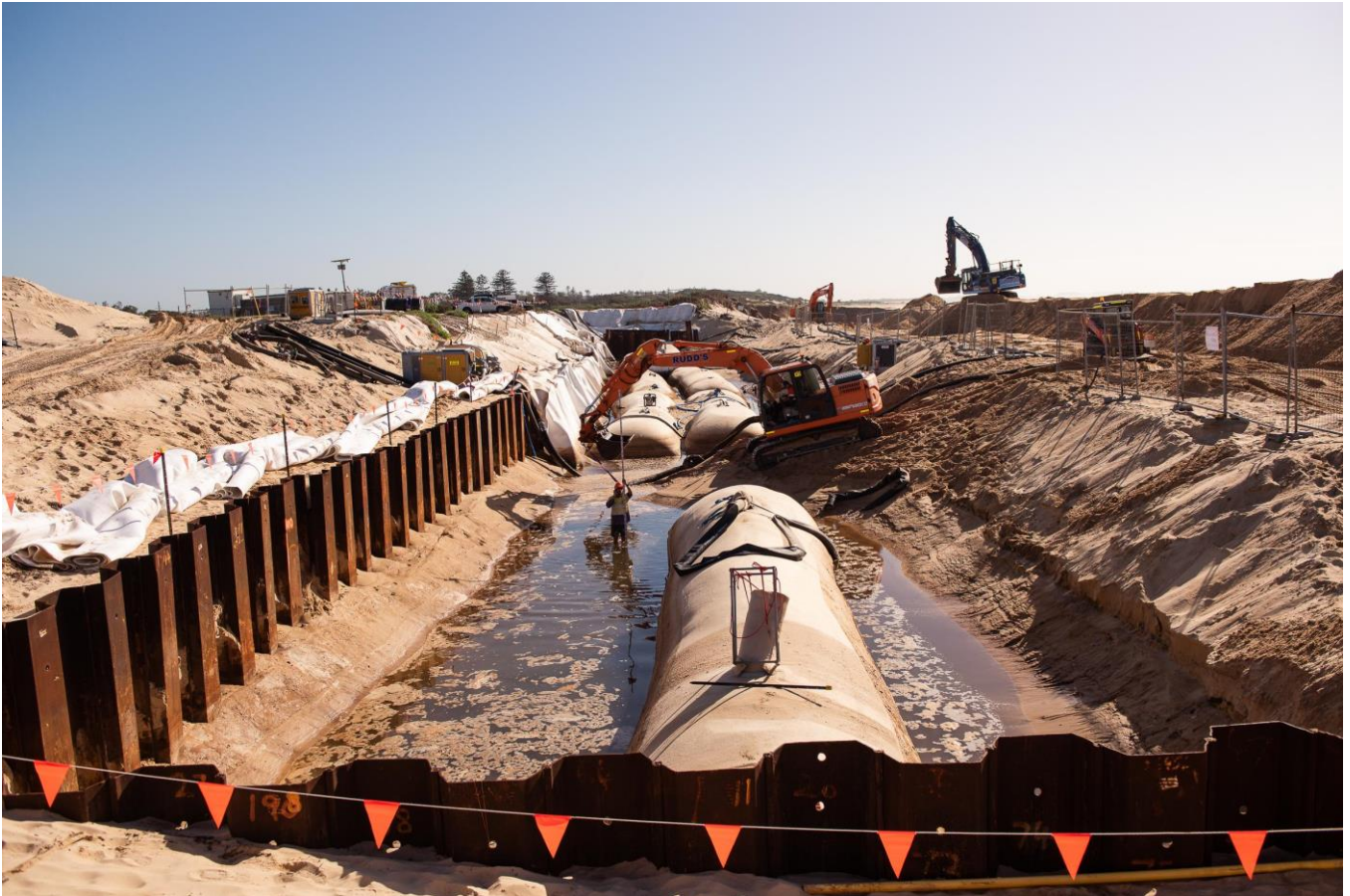
Image 3: Stockton site – Installation of mega container footing to protect landfill against future erosion
