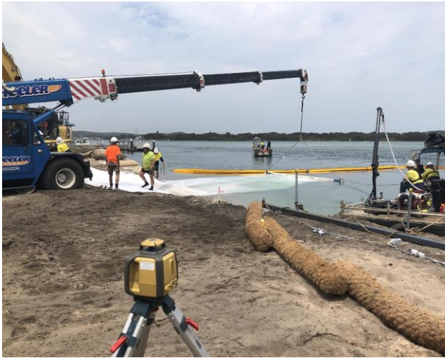
Figure 19: Deploying the first 'Lee bar' to hold geofabric underlying revetment and wrapping toe of structure water depths >5m
