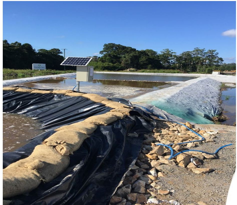
Figure 10 Another turkey nest HES basin installed in the northern Mooloolah River floodplain for dewatering and treatment of contaminated water from upstream sources.
