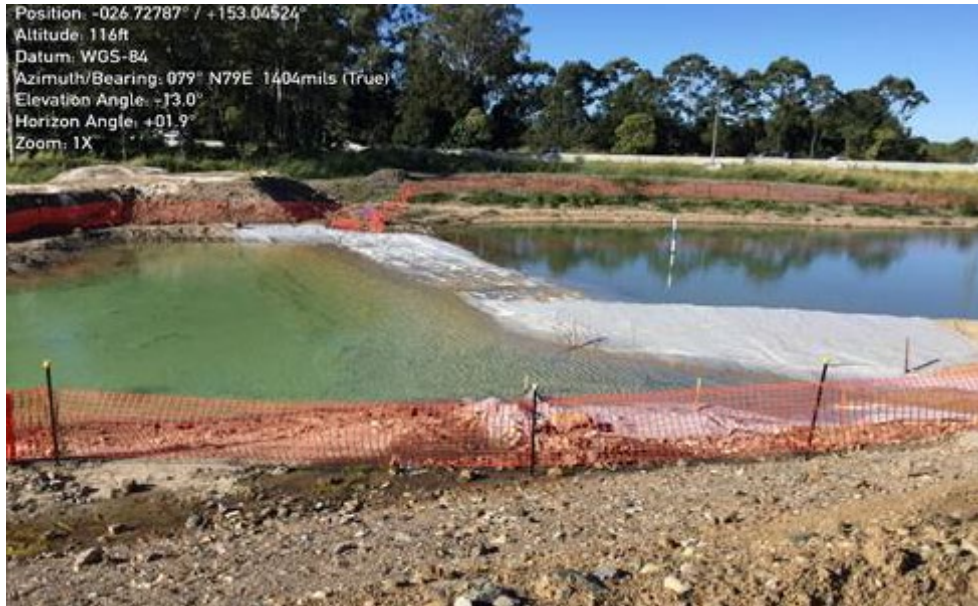
Figure 14 The HES basin in the northern work zone manages water received from multiple sub-catchments
