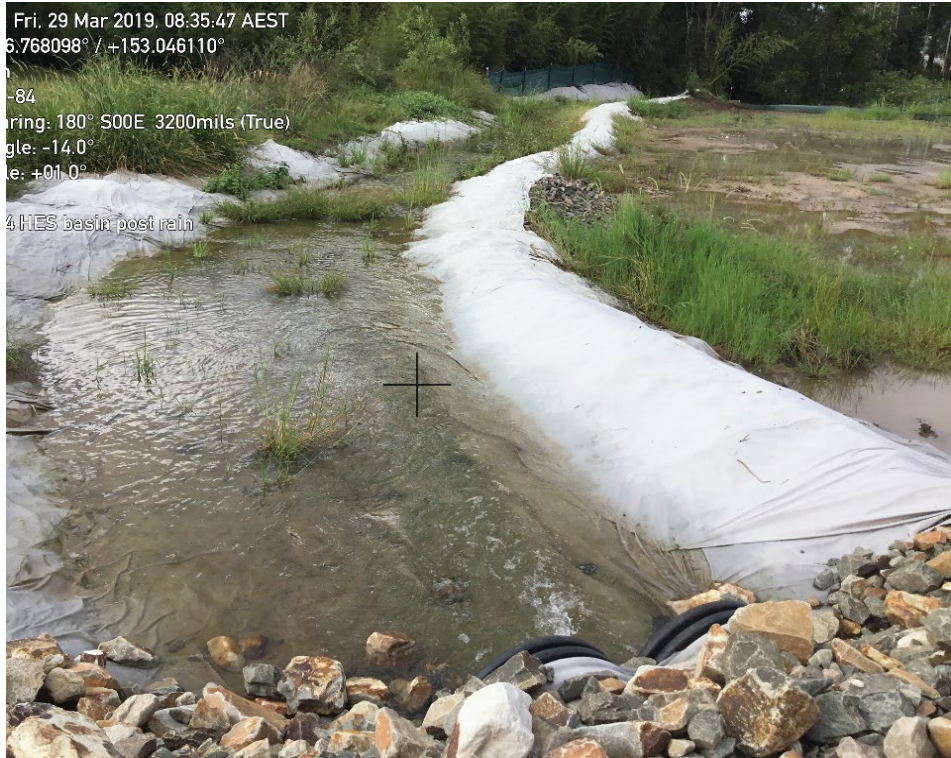
Figure 13 Water being discharged from the construction site shows following a 150mm rain event into the sensitive Mooloolah River catchment a distinct improvement after being treated in the HES basin.
