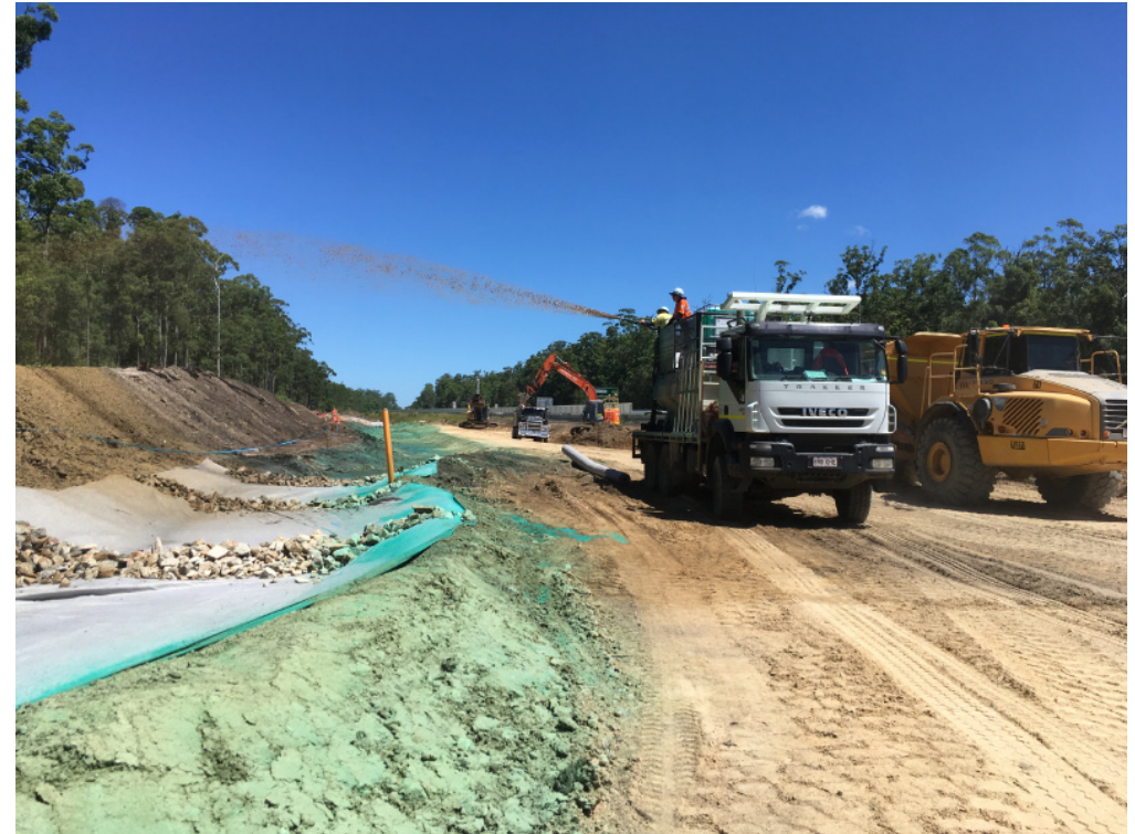
Figure 17 Dustbloc is used on site as an effective way of aiding soil stabilisation.
