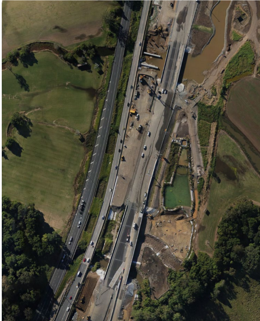
Figure 11 An aerial view showing the location of the HES basin in relation to the project works.
