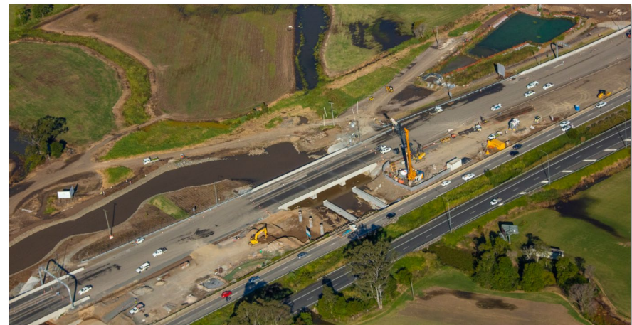
Figure 2 An innovative application of HES basins on site has managed ESC in challenging site conditions and effectively treated large volumes of contaminated water from upstream sources.
