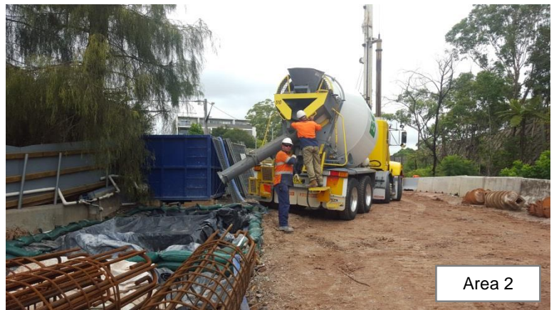
Photo 41: Concrete washout set up and positioned away from Cockle Creek, with sandbag bunding and plastic lining
