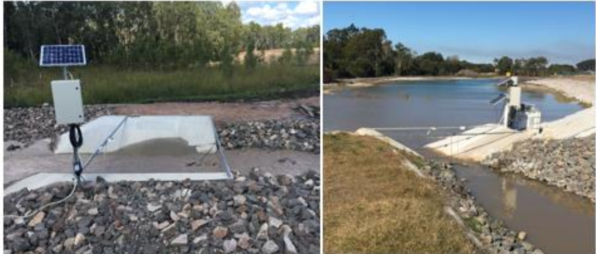
Figure 4.1.1 - Runoff entering HES basin (H6 left and H3 right) through concrete inlet. Monitoring equipment records inflow water quality data, and an automated dosing system provides treatment.
