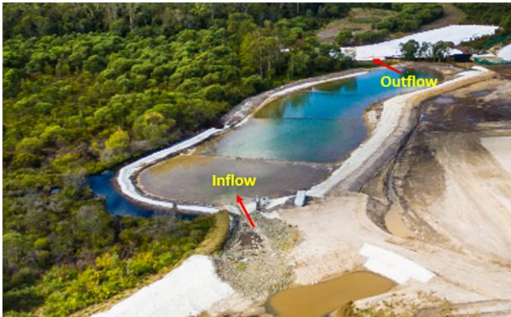
Figure 2.1.1 - HES Basin H3 displaying water quality and incorporating water sensitive urban design principles
