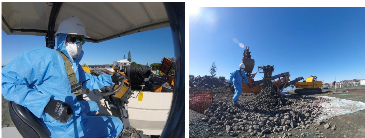
Full PPE during handling of Hazardous Materials. Uncomfortable in the heat to say the least. A challenge for workers
