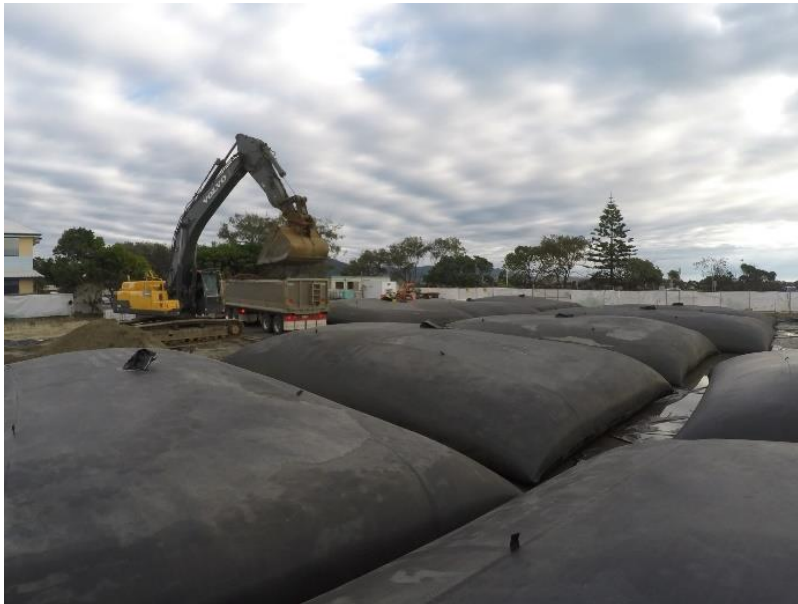
Geosynthetic Bags filled with contaminated sediment after de-watering being loaded out to waste management facility.
