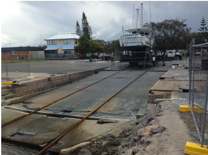
100Tn Coffs Harbour Slipway with Vessle prior to works. Note the drainage pits in the foreground that go under during high tide.
