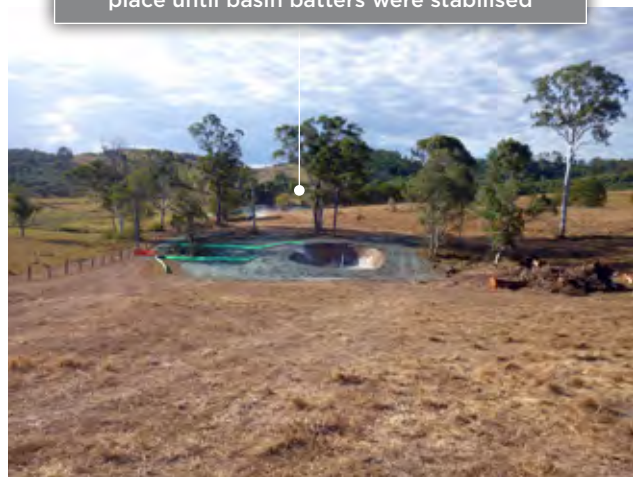
Sediment basin installation prior to clear and grub, with downstream Type 3 controls in place until basin batters were stabilised
