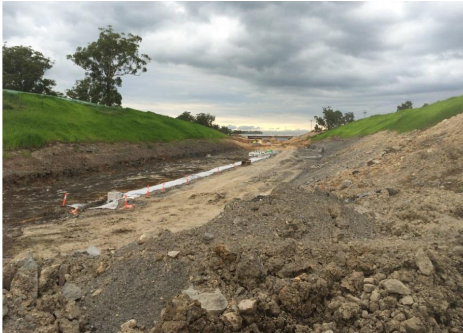
Progressive stabilisation with vegetated batters at Cut 6 during earthworks and drainage phase.
