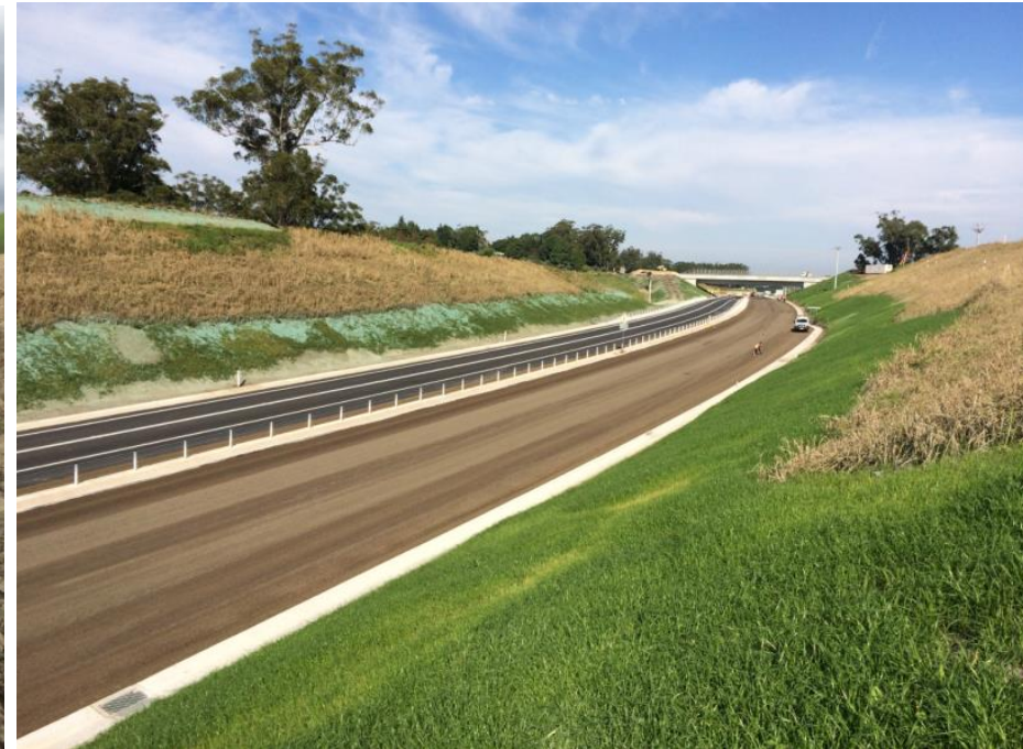
Fully stable batters at Cut 6 as pavement and finishing works are performed.
