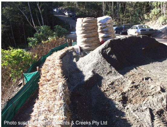
Photo 7 – Straw bales used to prevent stockpiled material shifting onto the sediment fence
