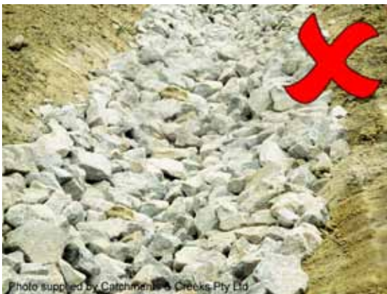
Poorly placed rock
