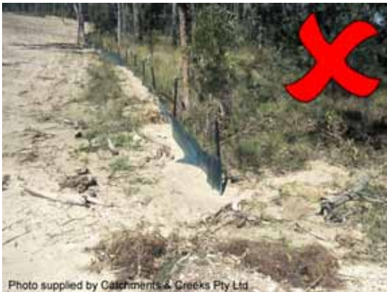
Fence not returned up-slope at end
