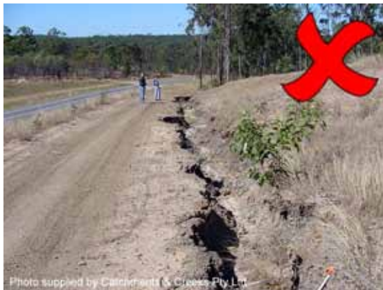
Severe erosion associated with catch drain cut into dispersive soil
