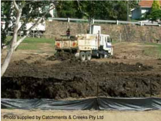
Truck bogged in wet soil
