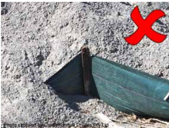
Sediment fence in need of maintenance
