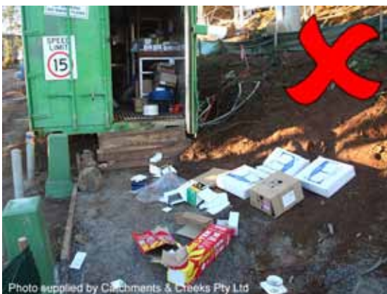
Poor litter control
