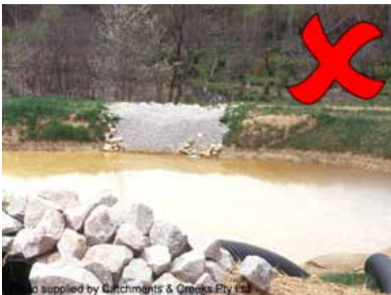
Inappropriate spillway crest profile
