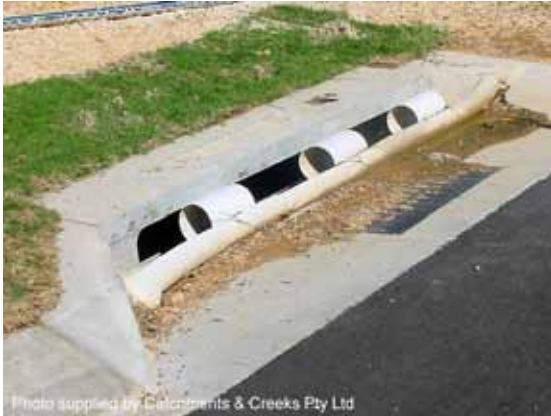
Photo supplied by Catchments & Creeks Pty Ltd Sag inlet sediment trap
