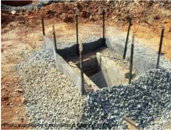
Mesh & aggregate drop inlet protection
