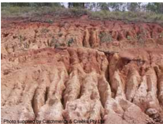
Erosion of a dispersive soil
