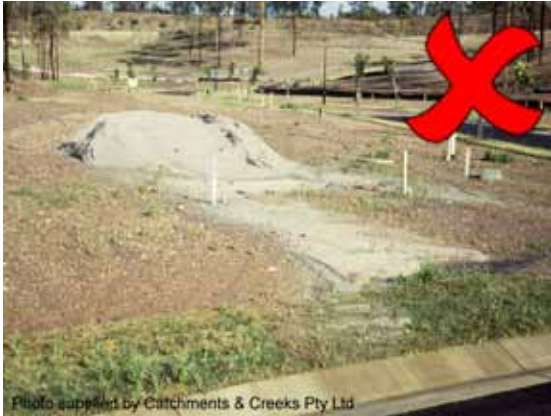
Inappropriately located sand stockpile
