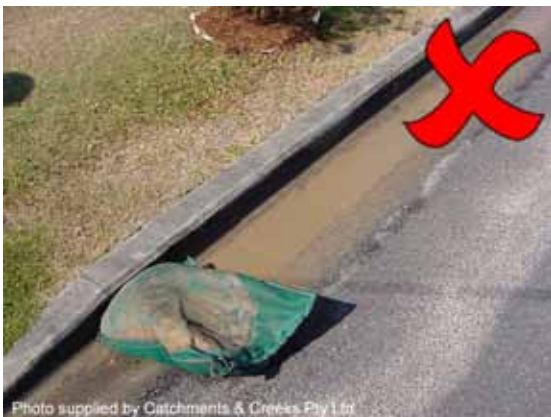
Photo supplied by Catchments & Creeks Pty Ltd Insufficient sediment control
