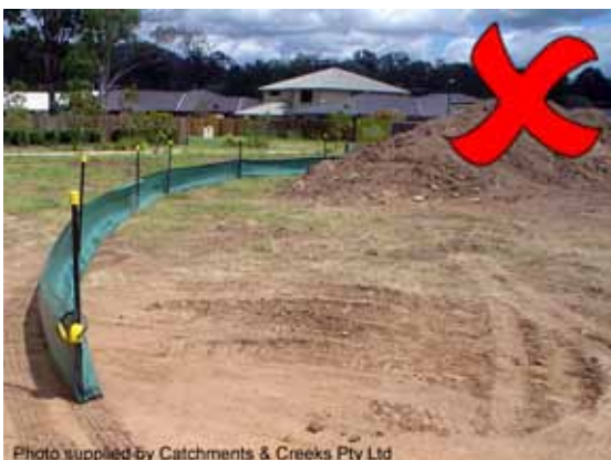
Post placed on wrong side of fence
