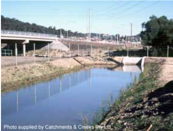
Sediment basin – wet basin
