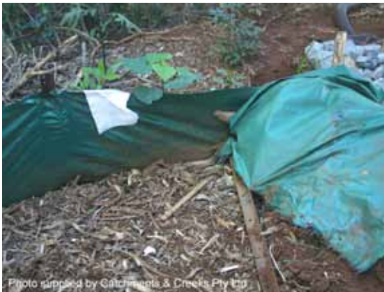
Damaged fence tagged for repair
