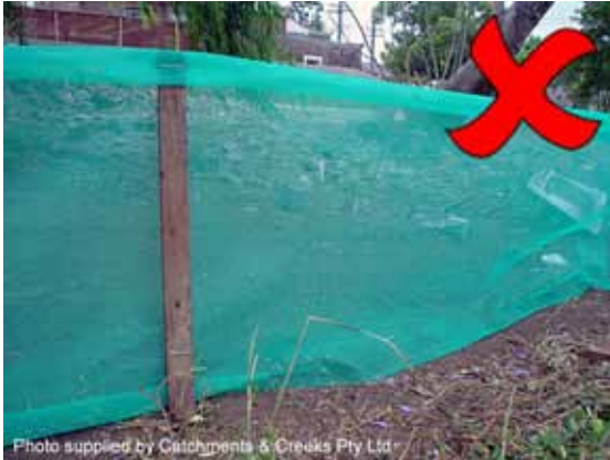
Inappropriate use of shade cloth
