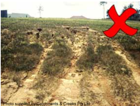
Damage to access road
