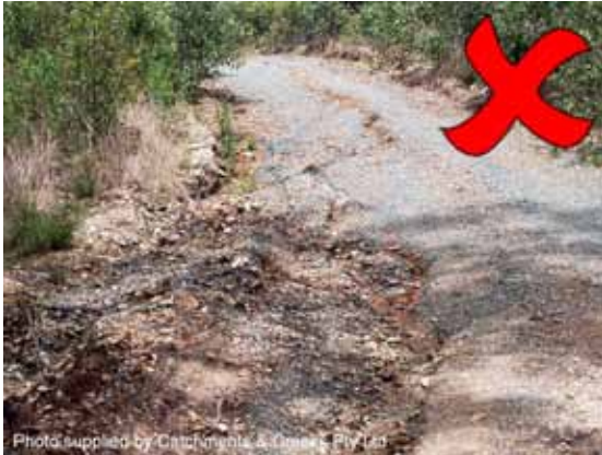
Inadequate drainage and erosion controls
