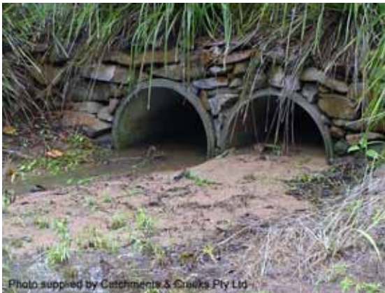
Sedimentation of drainage pipes
