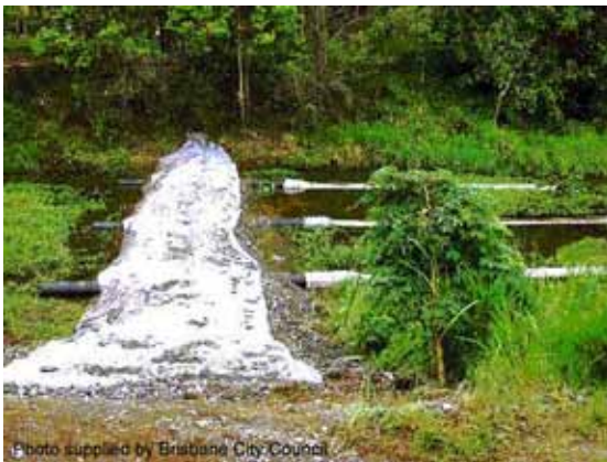
Instream sediment control system
