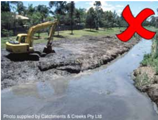
Inappropriate earthworks practice
