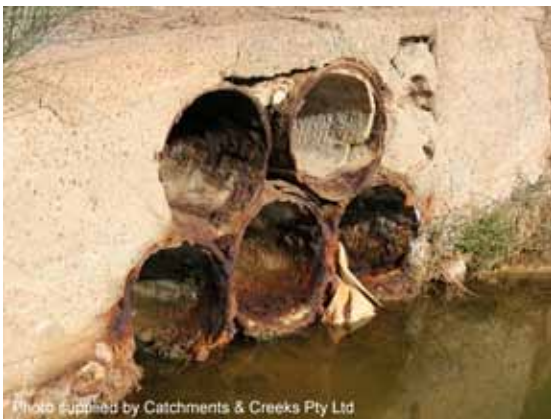
Culvert damage resulting from the exposure of acid sulfate soils
