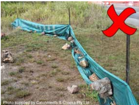
Toe of fabric incorrectly anchored
