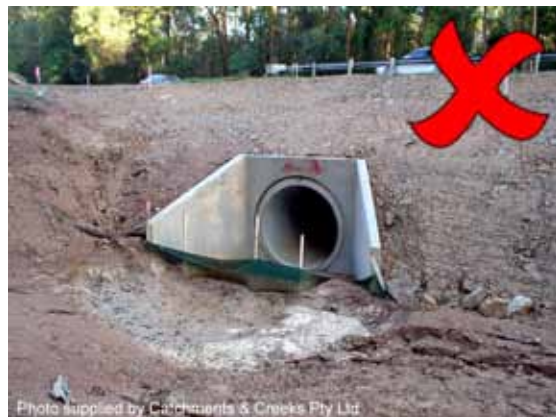
Inappropriate sediment control
