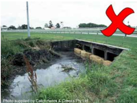
Inappropriate sediment control
