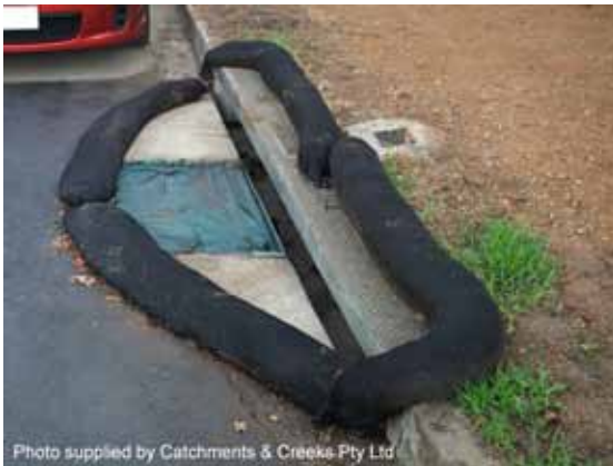
Photo supplied by Catchments & Creeks Pty Ltd Sag inlet sediment trap
