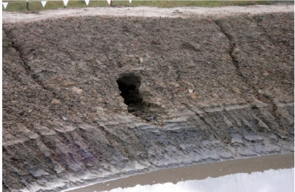
Tunnel erosion through a sediment basin wall constructed from dispersive soil
