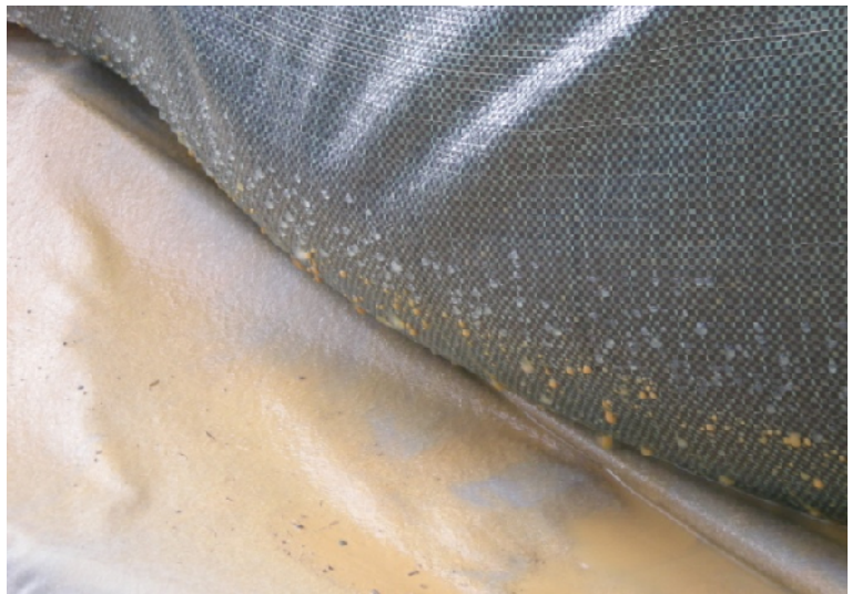
Turbid water seeping through a woven sediment fence
