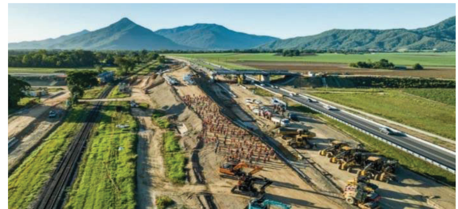
Figure 1: The Bruce Highway, Cairns Southern Access Corridor (Stage 3) - Edmonton to Gordonvale Project (E2G) is the largest infrastructure project delivered in Far North Queensland (Image: HSA Group)
