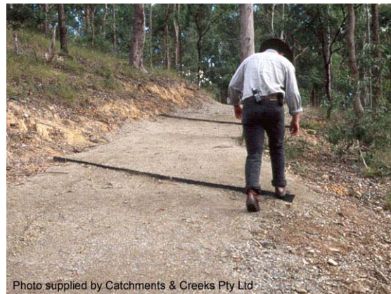
Photo 14 – Rubber strips used to direct stormwater of an outfall fire trail
