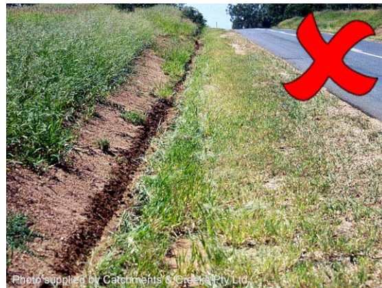
Photo 32 – Damage to toe of cut batter caused during road maintenance
