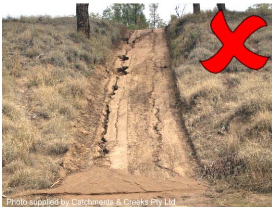
Photo 3 – Access roads cut into dispersive soil can experience severe erosion
