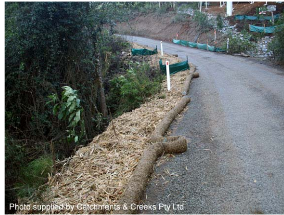
Photo 8 – Rehabilitation of eroded earth batter caused by unstable outfall drainage
