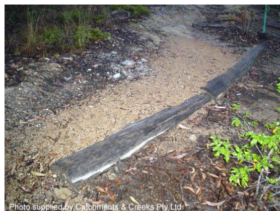
Photo 16 – Timber flow spreader
