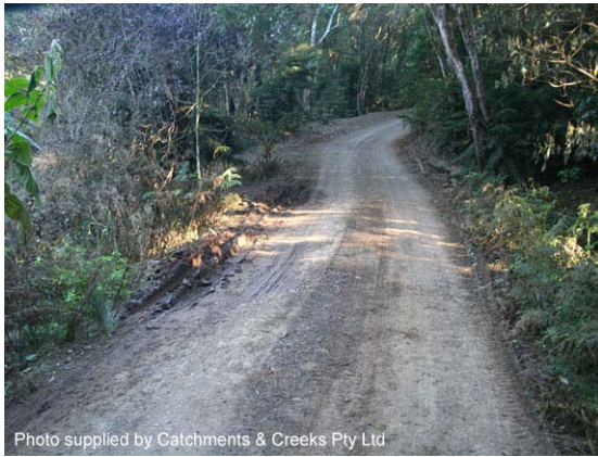
Photo 7 – Boggy ground formed on the edge of a road with outfall drainage
