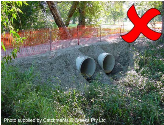
Photo 25 – Using only fine aggregate to form the fill embankment can result in severe wash-outs if overtopped
