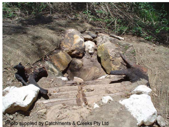
Photo 12 – Cross-bank discharge structure releasing flow down a steep slope
