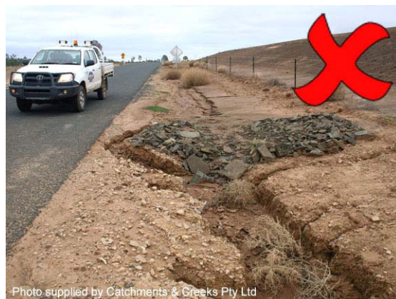
Photo 4 – Table drains cut into dispersive soil need to be treated and/or sealed with non-dispersive soil
