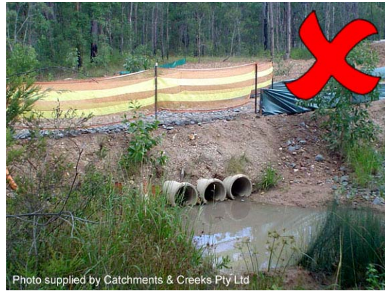
Photo 26 – If the culvert has insufficient hydraulic capacity, then overtopping flows are likely to cause severe bank erosion
