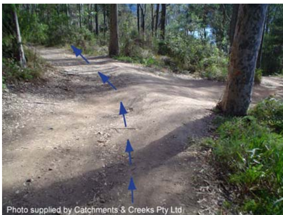
Photo 19 – Flow diversion bank (cross bank) at the crest of a descending road
