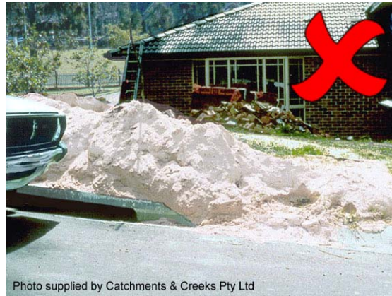
Photo 10 – Stockpiles of sand and other erodible materials must not be placed on the road verge or near stormwater inlets
