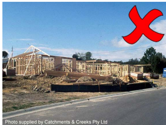
Photo 6 – Limited site access should not be used as an excuse to move building activities and stockpiles onto the footpath
