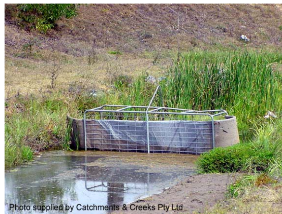
Photo 2 – Sediment cage in operation
