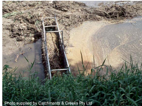
Photo 4 – Sediment filter cage
