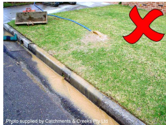
Photo 2 – Pumped inflow should not be released as concentrated flow onto a grass filter bed
