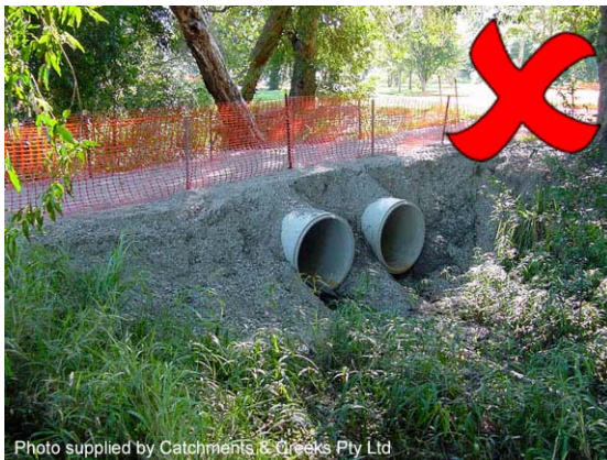
Photo 3 – Using only fine aggregate to form the fill embankment can result in severe wash-outs if overtopped
