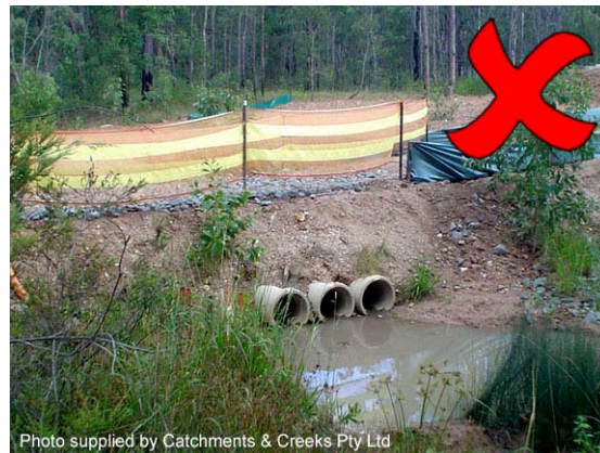
Photo 4 – If the culvert has insufficient hydraulic capacity, then overtopping flows are likely to cause severe bank erosion
