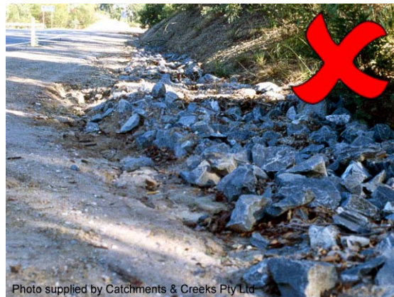
Photo 6 – In this example, placement of the rock has resulted in the rock-lined table drain being higher than the road shoulder
