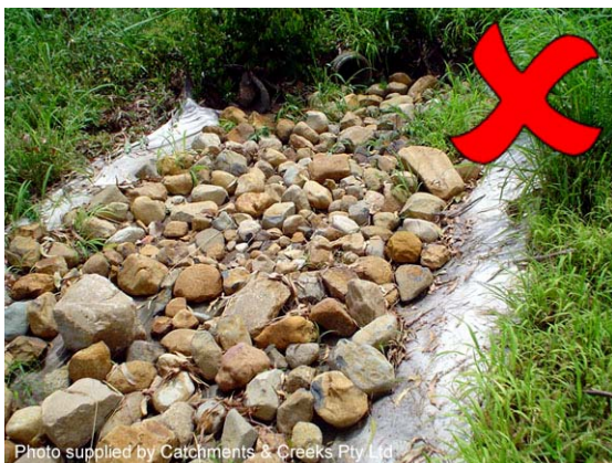
Photo 7 – Rounded rock can be significantly less stable than angular, fractured rock, especially when placed on steep slopes
