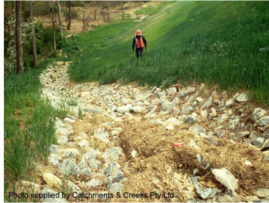
Photo 4 – Note how runoff from the adjacent batter is able to spill freely into the drain
