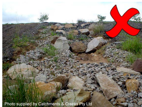
Photo 24 – Placement of a few large, anchor rocks down a steep slope will not help stabilise adjacent, under-sized rocks, and will likely cause flow diversion
