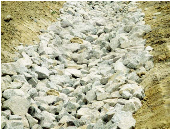
Photo 21 – Placement of the rock on the soil can result in erosion problems if significant lateral inflows occur
