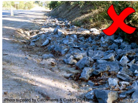
Photo 22 – In this example, placement of the rock has resulted in the rock-lined table drain being higher than the road shoulder
