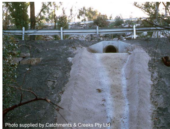
Photo 10 – Permanent concrete-lined batter chute
