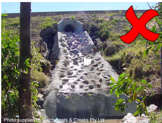
Photo 7 – Severe erosion along edge of chute caused by water spilling out of the chute
