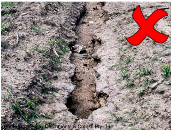
Photo 5 – Upper limit of erosion within a catch drain
