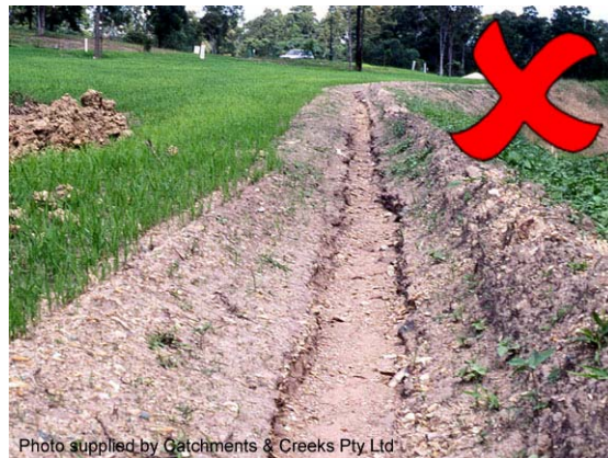
Photo 6 – Velocity-induced bed scour within a catch drain
