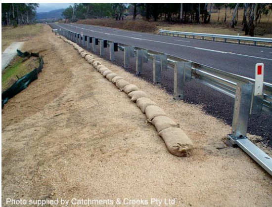
Photo 1 – Flow diversion berm used to minimise road runoff flowing down a steep, unstable section of the embankment
