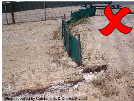
Photo 8 – If the ends of the fence are lower than the spill-through weir, then flows will bypass around the sediment trap causing erosion (as above)
