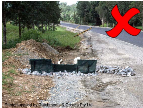
Photo 7 – Clearly, this sediment trap will not allow adequate ponding, and the shape of the structure prevents the spill-through weir from being functional
