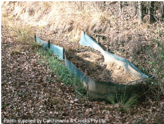
Photo 5 – U-shaped sediment trap within a steep table drain
