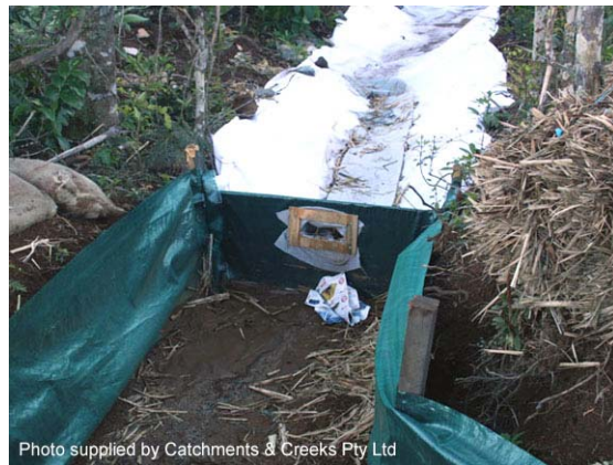
Photo 4 – U-shaped sediment trap incorporating a filter tube and geotextile outlet chute (note the sediment trap is formed from impervious plywood panels covered in fabric)
