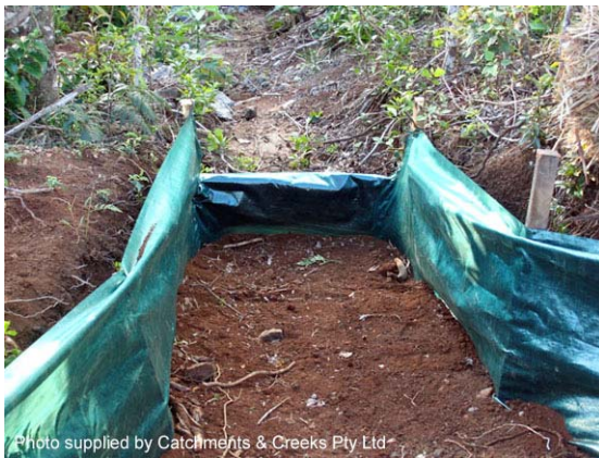
Photo 3 – Up-slope ends of the fence are flared out to adequately capture the inflow
