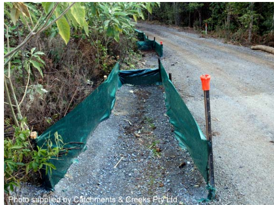
Photo 6 – U-shaped sediment trap within a mild-sloping table drain
