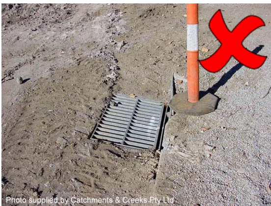
Photo 17 – No sediment control
