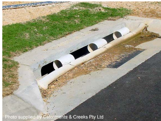
Photo 14 – Kerb inlet control system
