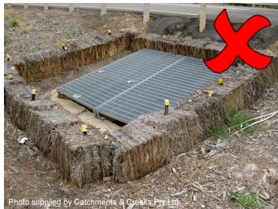
Photo 16 – Straw bale barriers are rarely adequate sediment traps
