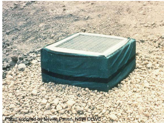
Photo 6 – Fabric drop inlet protection
