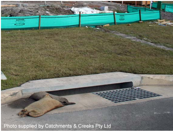
Photo 11 – On-grade kerb inlet control
