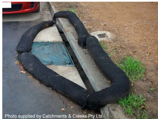
Photo 4 – Filter sock sag inlet sediment trap (supplementary system)
