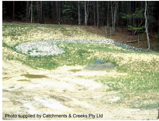
Photo 16 – Emergency spillway located within virgin soil to the side of the embankment
