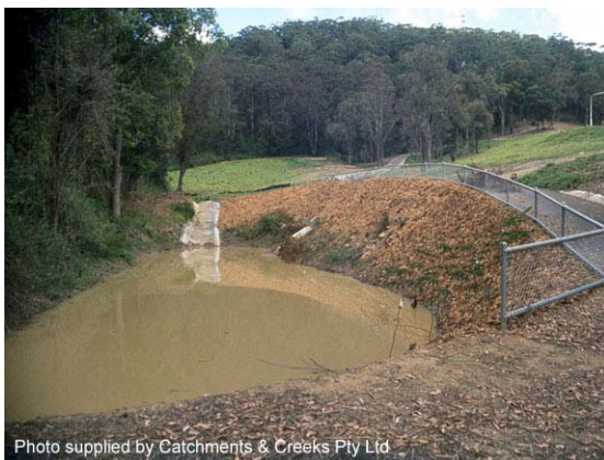
Photo 21 – Sediment basin with poor access for de-silting operations
