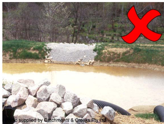
Photo 20 – Spillway crest with inadequate depth or profile
