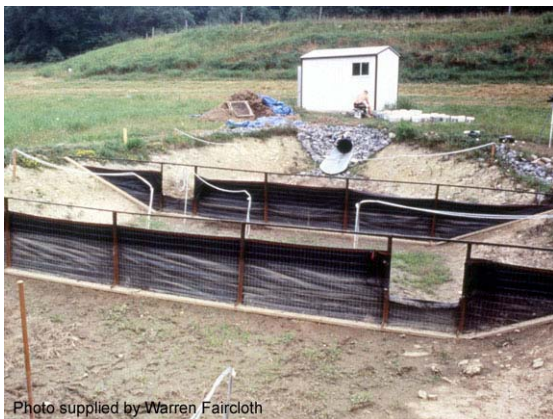
Photo 3 – Inlet chamber can also act as mixing chambers for the addition of flocculants
