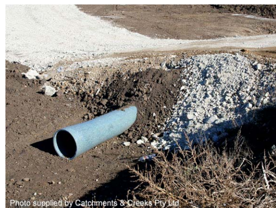
Photo 6 – Pipe to pass up-slope runoff under a rock pad
