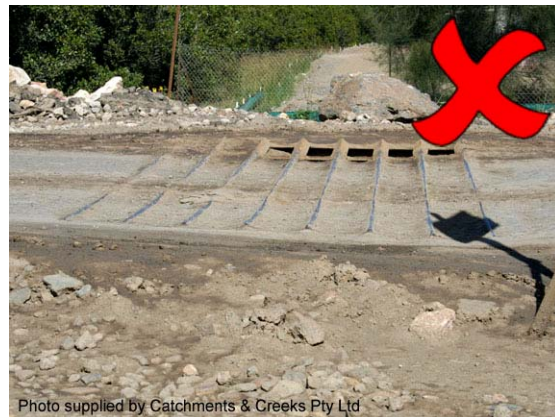
Photo 10 – Heavy sedimentation should not be allowed to occur at construction exits prior to their maintenance
