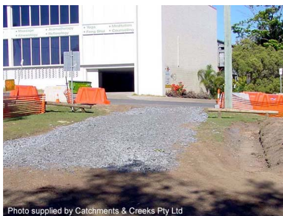
Photo 7 – Drain down-slope of rock pad directing sediment-laden runoff to a nearby sediment trap.
