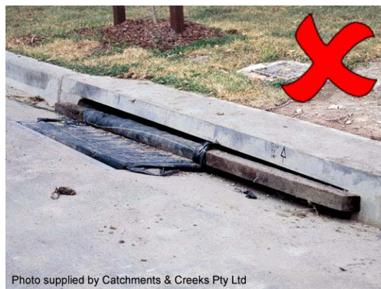
Photo 6 – An inappropriate sediment trap for an 'on-grade' kerb inlet
