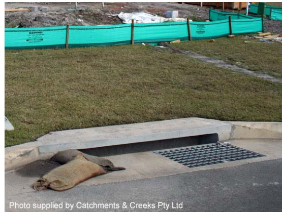
Photo 2 – On open roadways there may be strict limitation on how far the sandbags can extend into trafficable lanes
