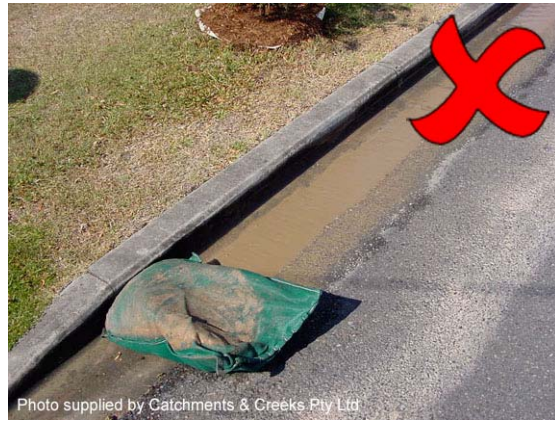
Photo 4 – One sandbag is usually not enough!
