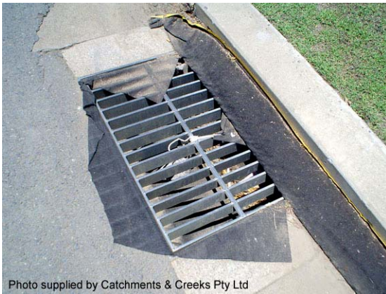
Photo 1 – Temporary gully bag
