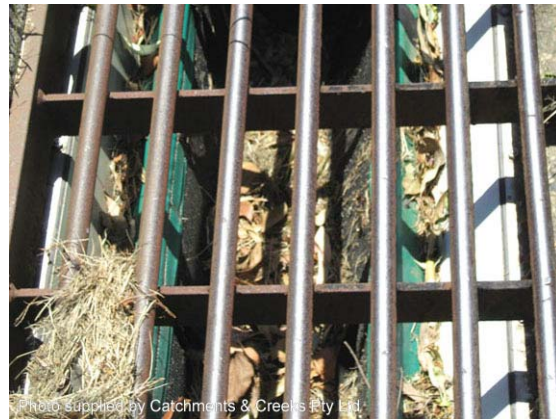
Photo 2 – Permanent gully bag
