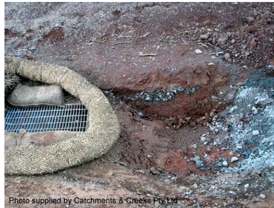
Photo 2 – Excavated drop inlet protection (poor example)
