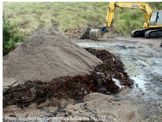
Photo 2 – Berm showing a breach point (centre) with flow passing over the berm
