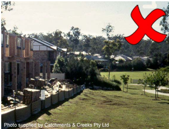
Wheel damage to buffer zone
