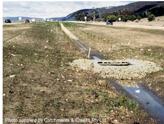
Photo 2 – Block and aggregate drop inlet protection placed around a drainage inlet within a dual carriageway median strip
