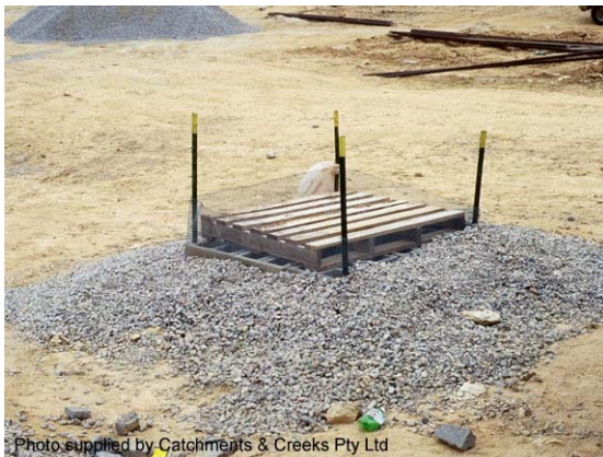
Photo 3 – Type A block and aggregate sediment trap (note, most blocks are turned upwards to prevent through-flow)
